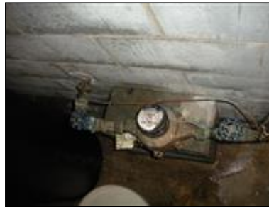
Main Water Shut-off
