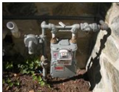
Main Natural Gas Shut-off
