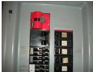
Main Electrical Shut-off
