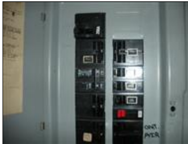
Main Electrical Shut-off
