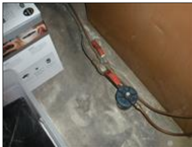
Main Fuel Oil Sweep Valves
